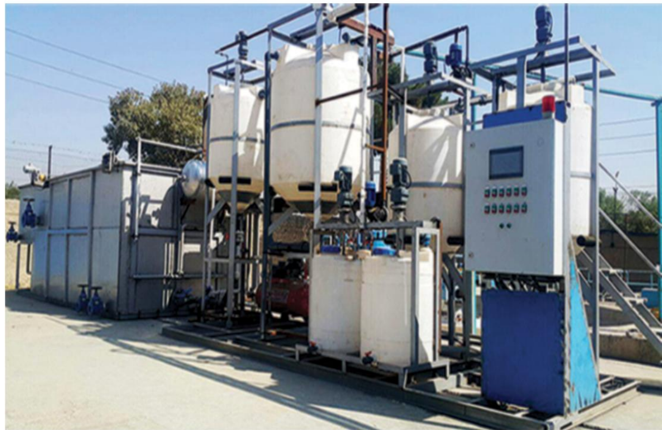
DAF Unit with coagulant and flocculate preparation & mixing sections, 30 m 3 /h waste-water feed
