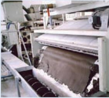
Municipal Sewage Sludge
