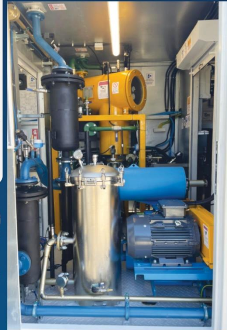
Purification Room (Vacuum Chamber, Cartridge Filter, Roots Blower, Demister, Charcoal Filter, Feed & Discharge Pumps, ...)
