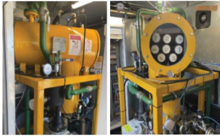
Vacuum Chamber consists of Coalescer Filters, Vacuum Pump & Booster for Removing Gas & Water from Oil
