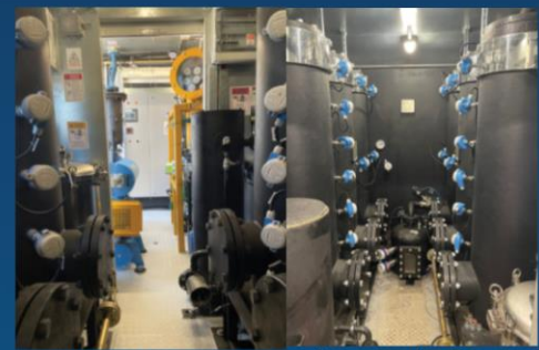
Plant in 3 Rooms
