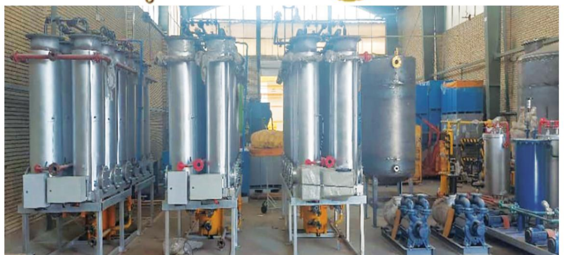
POLISHLUBE PLANT, 3 Bank, 36 Jacketed Reactors, Contains 6500 kg TURBOSORB Adsorbent, 15 ton/day
